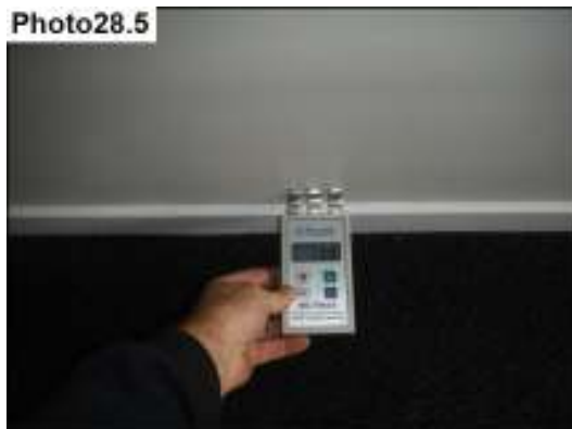
Photo28.5 Moisture reading behind cracked tile in the shower. 13.8%
