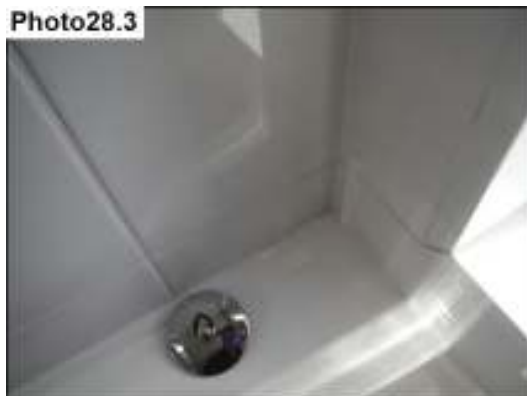
Photo28.3 Silicone sealant around the bath is starting to lift. This will need redoing soon.
