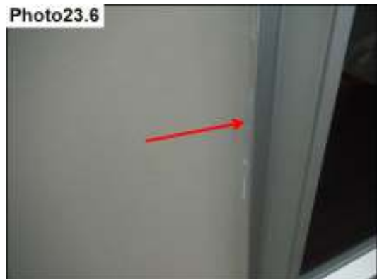
Window need to be resealed to the cladding when the house is painted.
