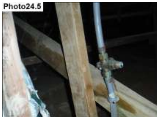
Leak in the pipe fitting next to the hot water tank.
