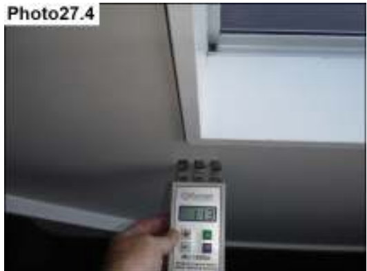
Moisture reading to the stairwell window. 11.3%
