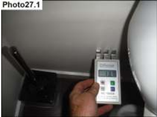
Moisture reading behind the down stairs toilet
