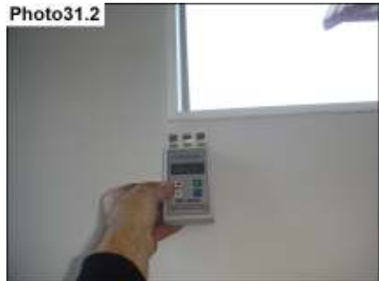
Moisture reading to the stairwell window. 14.3%
