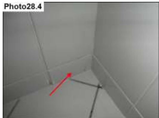
Photo28.4 Cracked tile in the shower. this needs attention.
