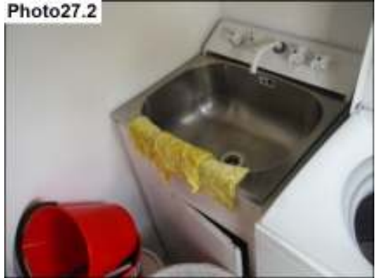
Supertub needs fixing to the wall.
