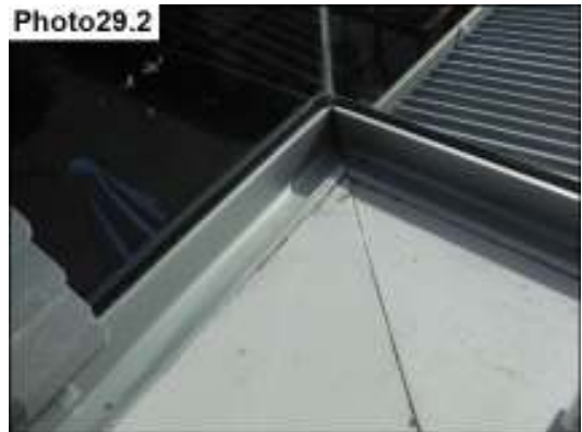
Condensation damage noted to some of the window sills.
