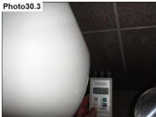
Moisture reading behind the master ensuite toilet. 11.6%
