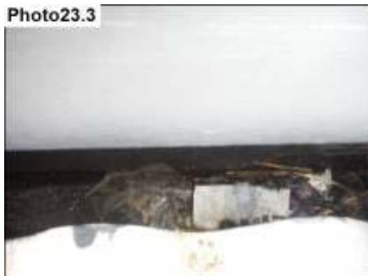
Debris in the internal gutter noted.
