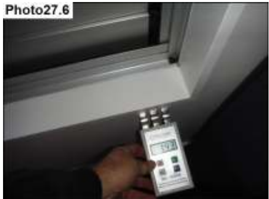
Moisture reading to bedroom 1 14.3%
