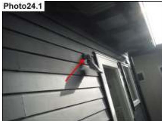
Outside light fitting is broken
