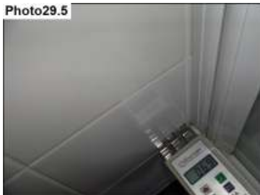
Moisture reading to the ensuite shower/bath. 6.9%
