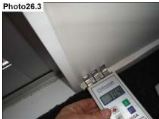
Moisture reading to the ranch slider from the second lounge area. 30.4%
