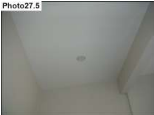
Smoke alarm need to be reinstalled.
