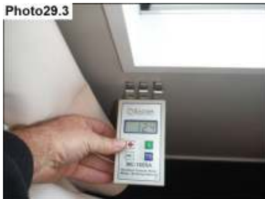
Moisture reading to bedroom 3 12.4%
