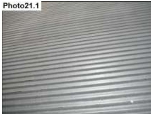
Roof area needs washing down
