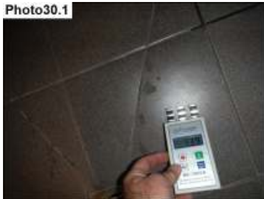
Moisture reading to the master ensuite shower. 13.9%
