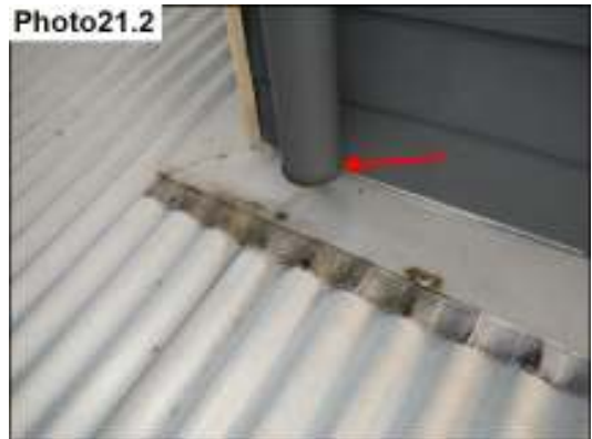
Recommend fitting spreader pipes to the bottoms of the down pipe.
