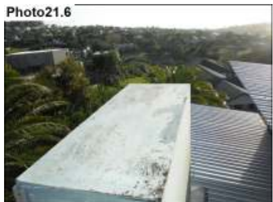
False chimney wasn't painted last time the house was. This needs attention.
