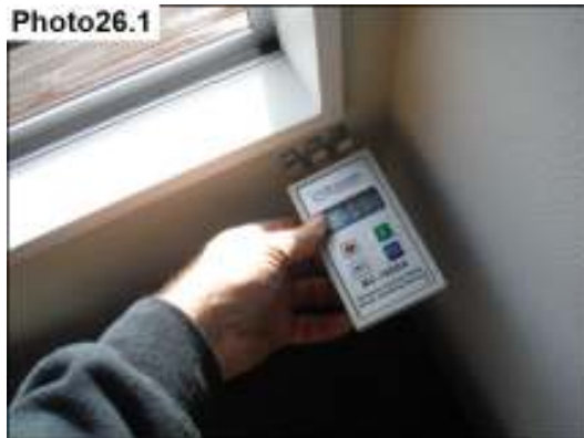
Moisture reading to the dining area. 9.0%
