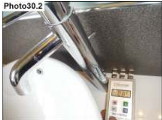
Moisture reading to the master ensuite basins. 8.5%
