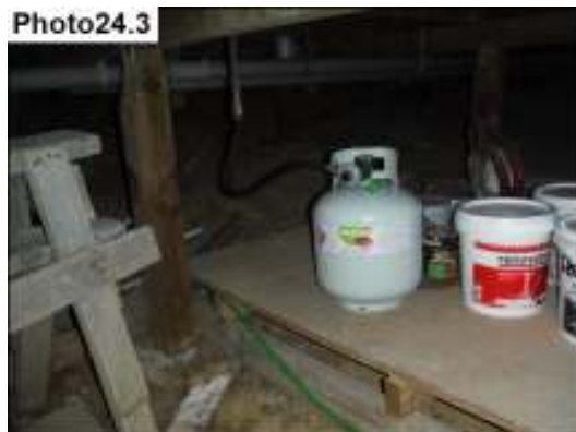
Gas bottle for the gas hob is under the house.
