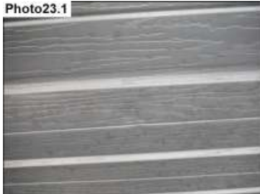
Dents noted in the garage door.
