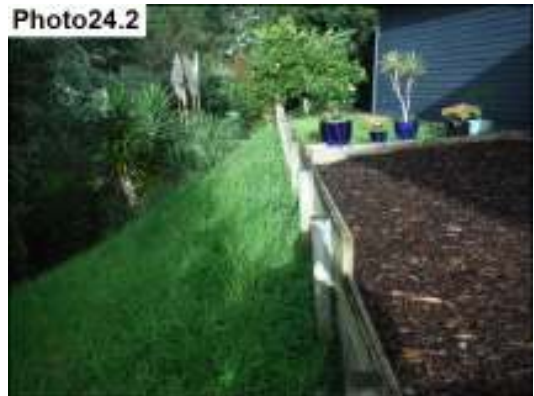
Movement noted to the rear timber retaining wall.
