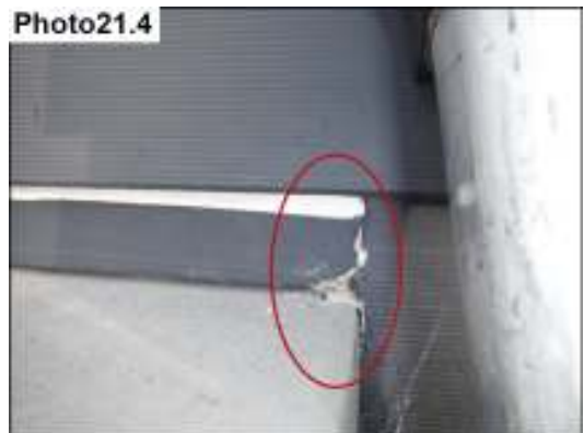
Cracking note to the weather board around some of the flashings.
