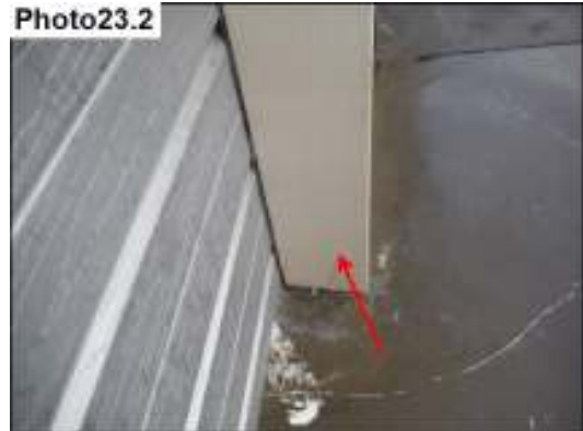
Garage door surround needs sealing and painting.
