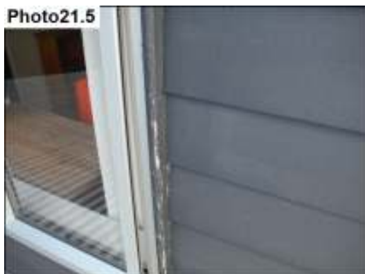
House will need repainting in the near future.
