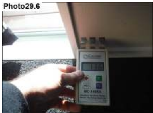
Moisture reading to the master bedroom. 13.6%
