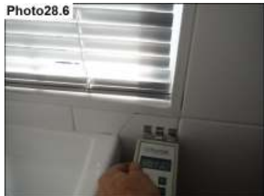
Photo28.6 Moisture reading at the cracked tile to the bath. 12.4%
