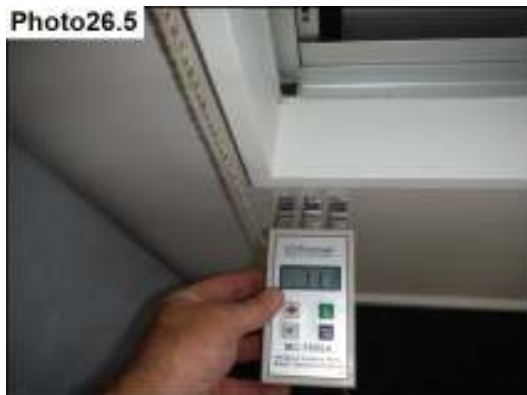
Moisture reading to the window in the second lounge. 11.1%
