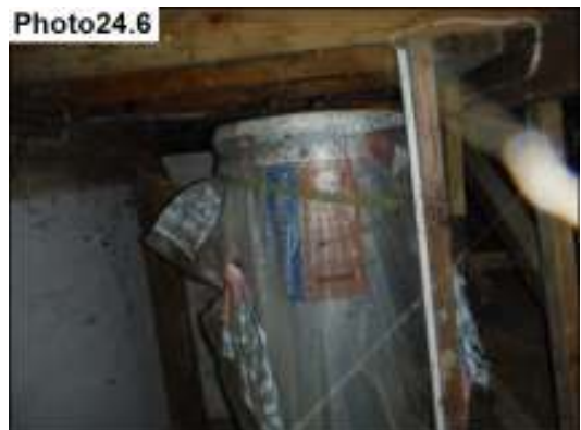
250 litre mains pressure hot water tank is under the house. Date stamped 02/2002
