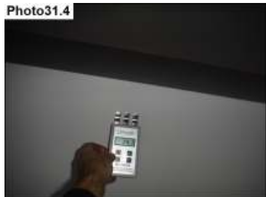
Moisture reading behind the internal gutter. 14.1%
