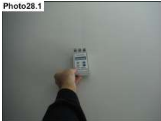
Photo28.1 Moisture reading to the crack in the wall in bedroom 1. 11.5%
