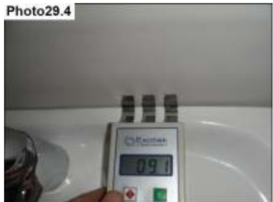
Moisture reading to the ensuite up stairs basin. 9.1%
